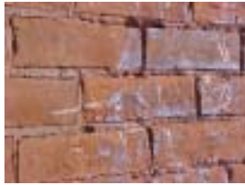
Brick and Mortar damage
