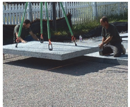
A pre-cast permeable concrete parking lot being laid on the UVM campus in Burlington. Photo credit: University of Vermont.
