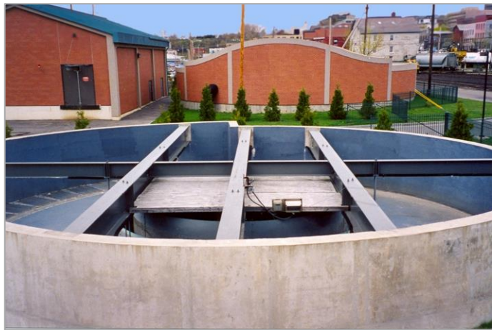
Vortex Swirl Separator at Main WWTP
