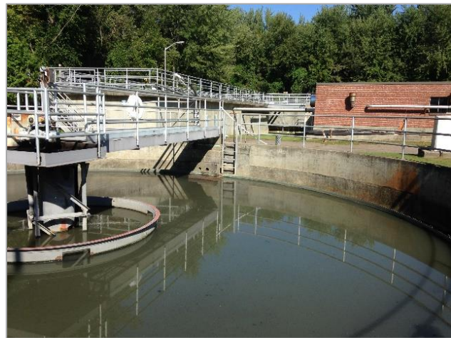
Clarifier at North WWTP
