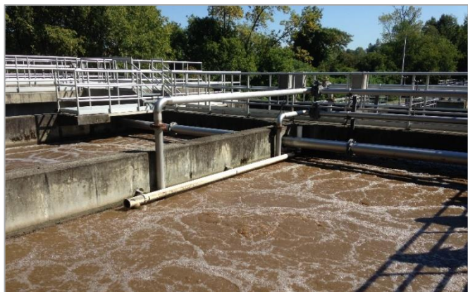
Aeration tanks at East WWTP
