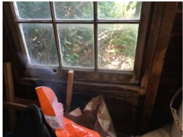
Moisture damage at window.
