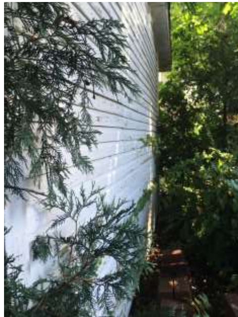
Back side of the siding bows outward.
