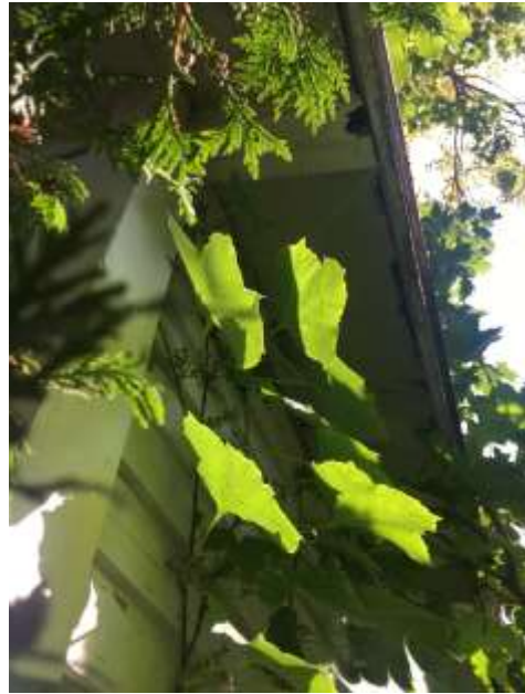
Deteriorating rafters & roof sheathing at South eaves.
