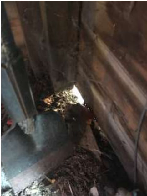
Northeast corner of structure sits above grade = no structural support.
