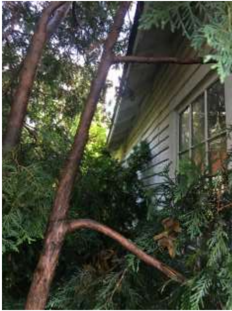
Two windows at rear (historic) section of structure & seam connecting historic to later addition.
