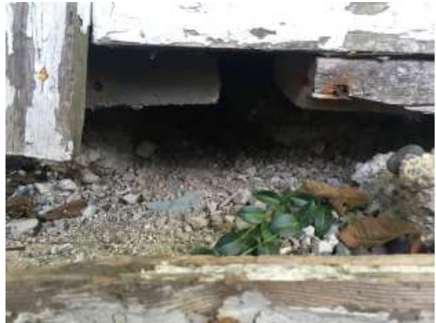
Northwest corner not setting on structural foundation. Gravel has washed out.
