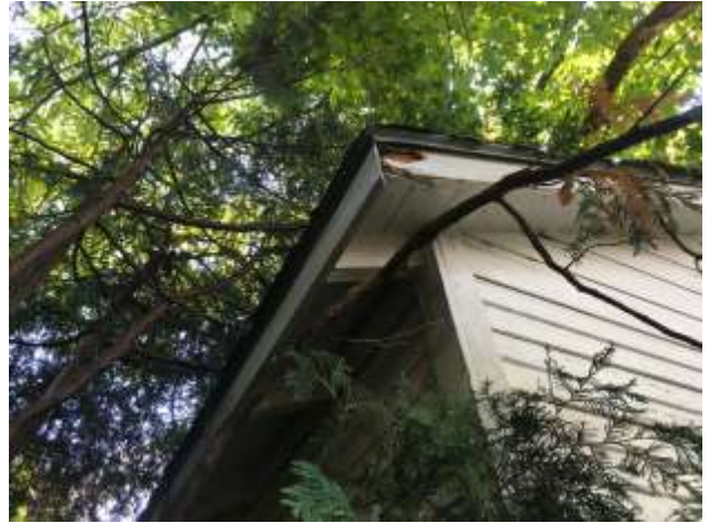
Deteriorated trim at roof eaves.
