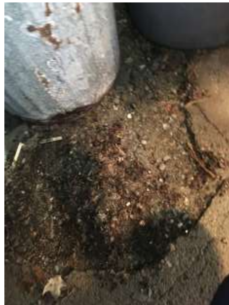
Deteriorated interior slab. Concrete appears to be a topping slab on gravel with no structural slab.
