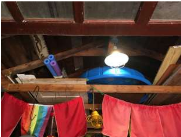
Moisture damage at roof and framing.
