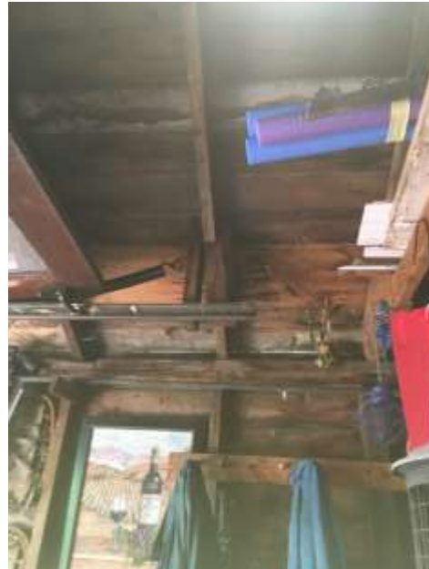
Moisture damage at roof and siding. Broken OHD track.
