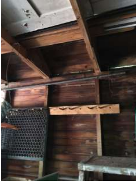
Moisture damage at siding- South wall.
