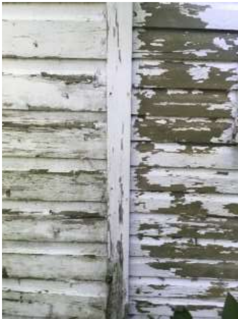
Deteriorating seam that separates the historic structure and the later addition.
