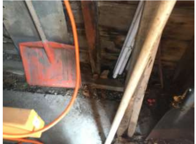
Gap between concrete slab and structure = structure sitting on grade with no structural support. Water damage at siding and framing.
