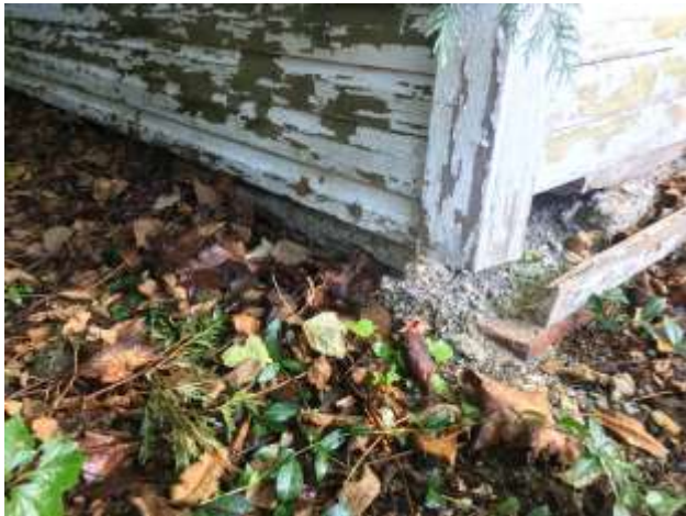
Northwest corner of structure floats above grade.
