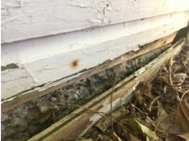
Southwest wall – previous concrete pour has pushed out the siding board at grade.
