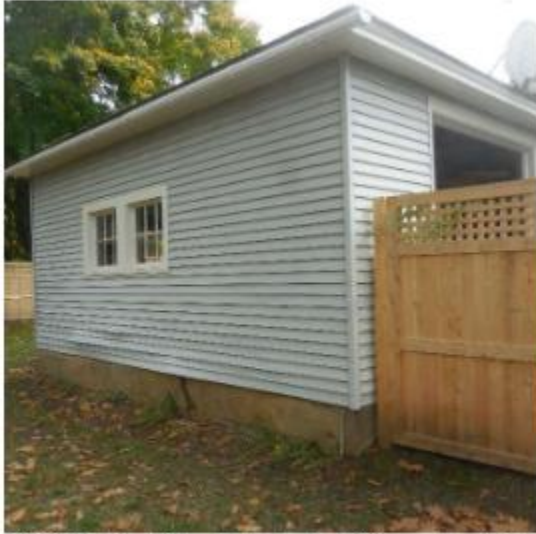
PHOTO 2: West Side - Note buckled siding and vertical crack in foundation/slab
