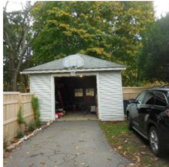
PHOTO 1: South Side - Note slight wacking of building to the left (west) side
