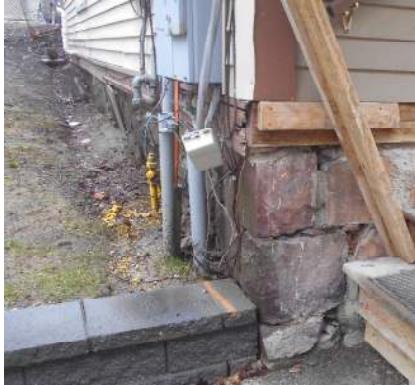
The north wall has pushed in several inches and does not appear stable. There are deteriorated mortar joints and drainage slopes back towards the building.
