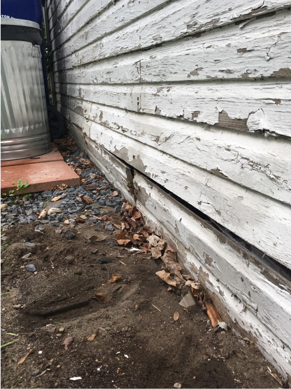
South side detail (deteriorating siding shifted during attempt to straighten structure)
