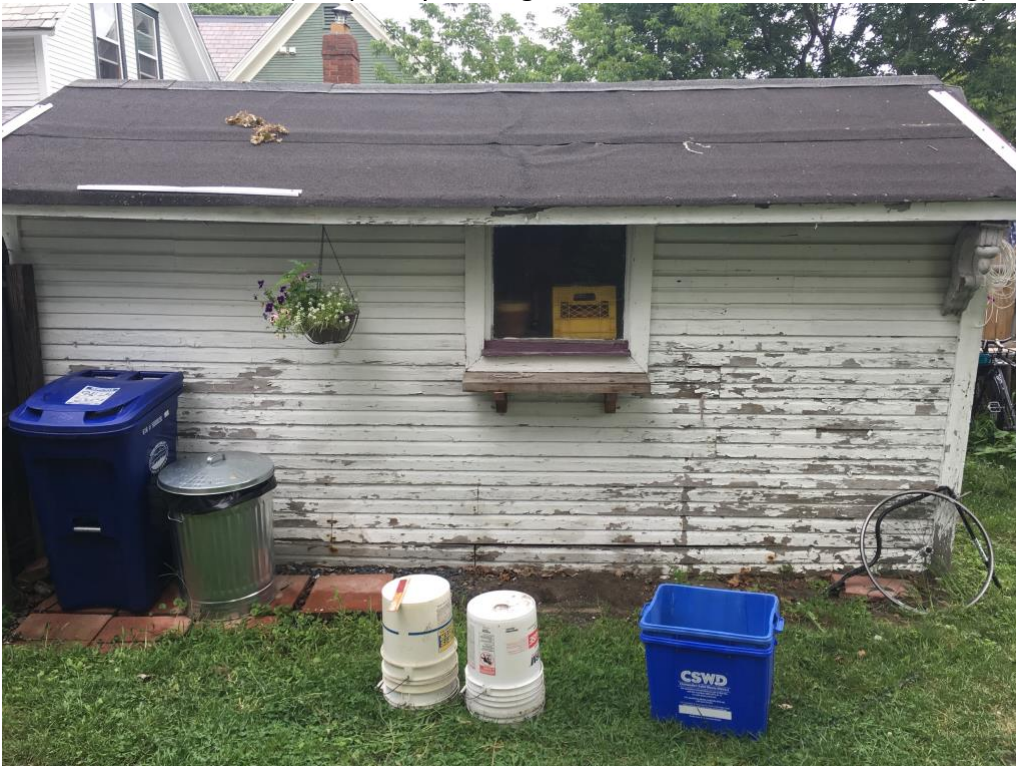
Shed from South side (temporary roofing added summer 2017 after leaking)
