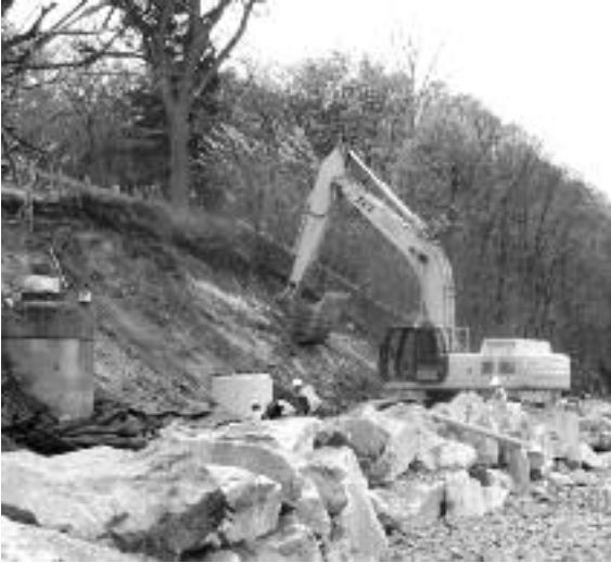
Construction to bolster the bike path near Lakeview Cemetery—this was one of the five bike path sections badly damaged in the May 2011 floods.
