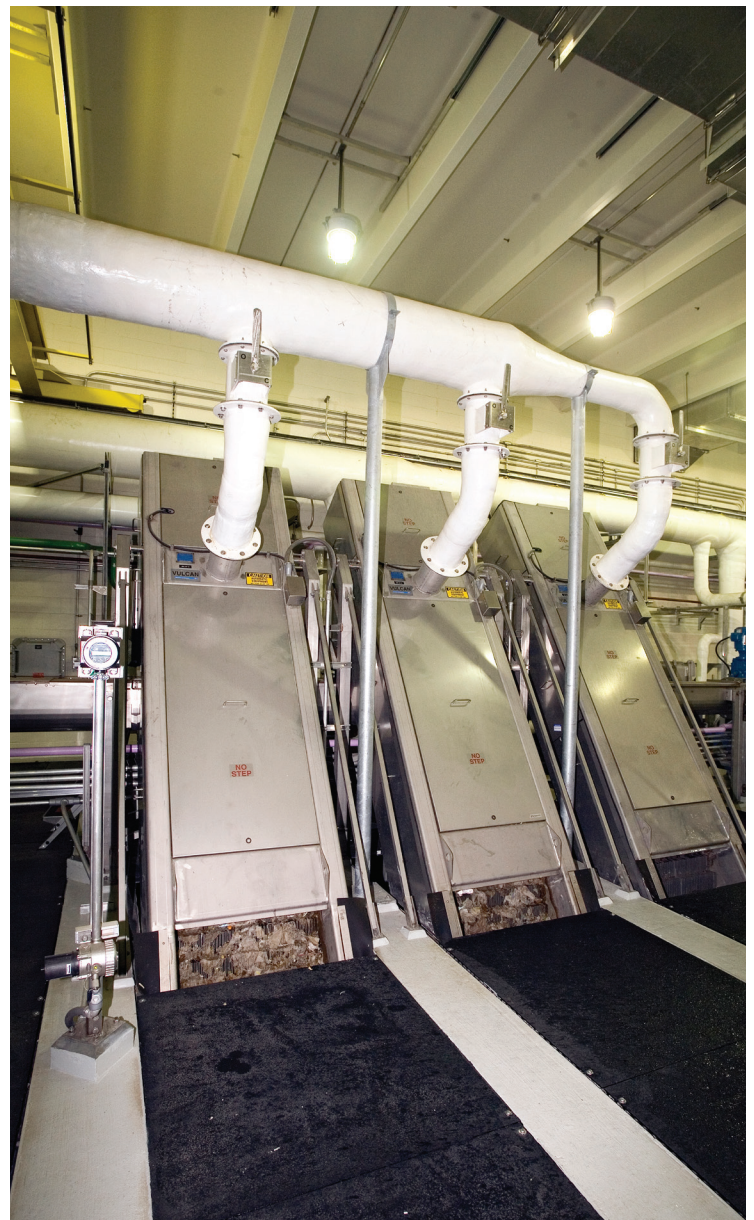
Large screens, like those shown here, are typically used to remove larger debris and other solid materials from wastewater as it enters a treatment plant.
